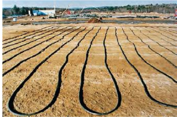
Fig. 7. A hydronic heating system installed under the slab and attached to the formwork [10].
