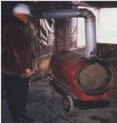
Fig. 6. Petroleum fuel-fired heater to maintain curing temperature in enclosed space [10].
