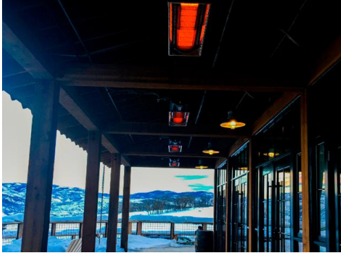
Fig. 9. Infrared heaters used for heating outside areas [12].
