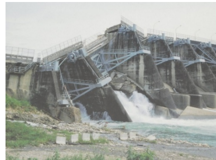
Fig. 2. Damage of the gravity concrete dam in the 1999 Chi-Chi earthquake (panel of the 921 Earthquake Museum of Taiwan).
