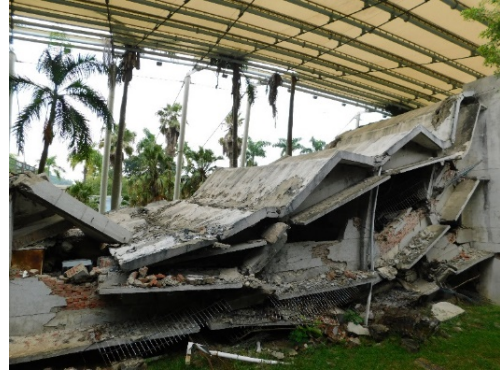
Fig. 4. Collapse of the Guangfu Junior High School building.
