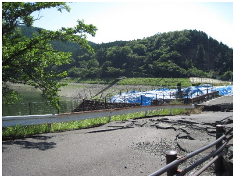
Fig. 1. Damage of the Oohata dam due to the fault displacement.
