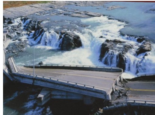
Fig. 5. Collapse of the bridge and waterfall due to the fault displacement (panel of the 921 Earthquake Museum of Taiwan).
