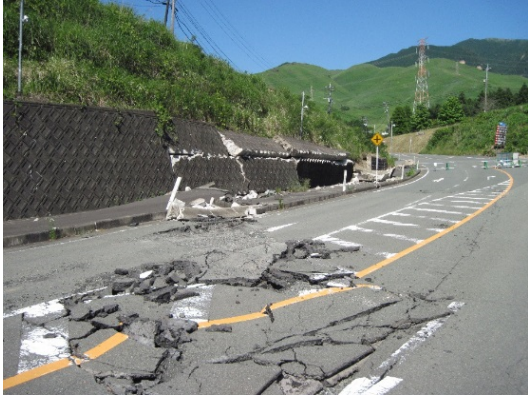
Fig. 7. Ground surface above the fault.
