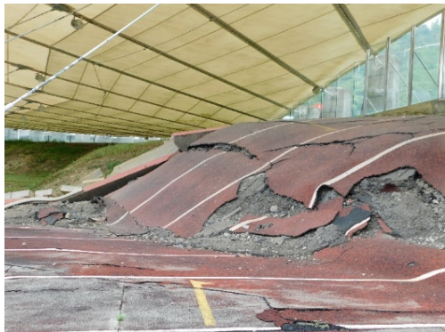
Fig. 3. Deformation of sports field due to fault deformation.
